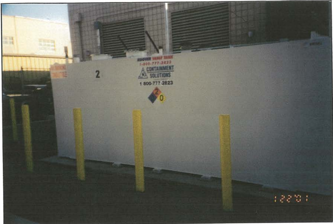
Generator #2 Fuel Tank B5
