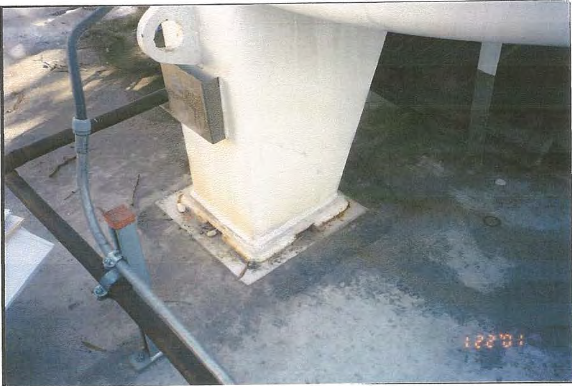
Oxygen Tank Anchorage C1
