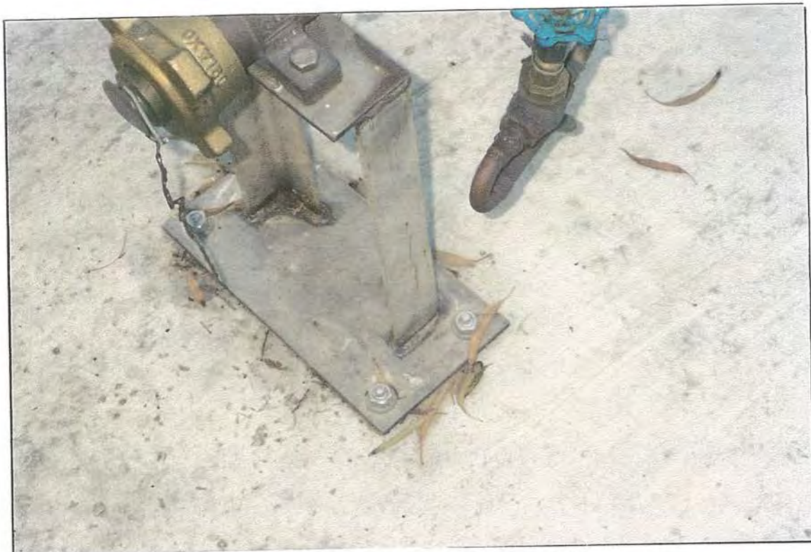
Oxygen Tank Anchorage C1
