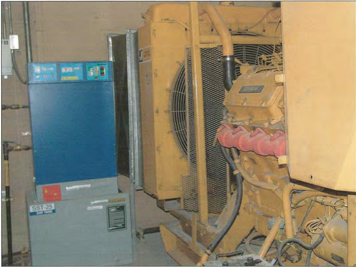
Generator #2 Day Tank B6
