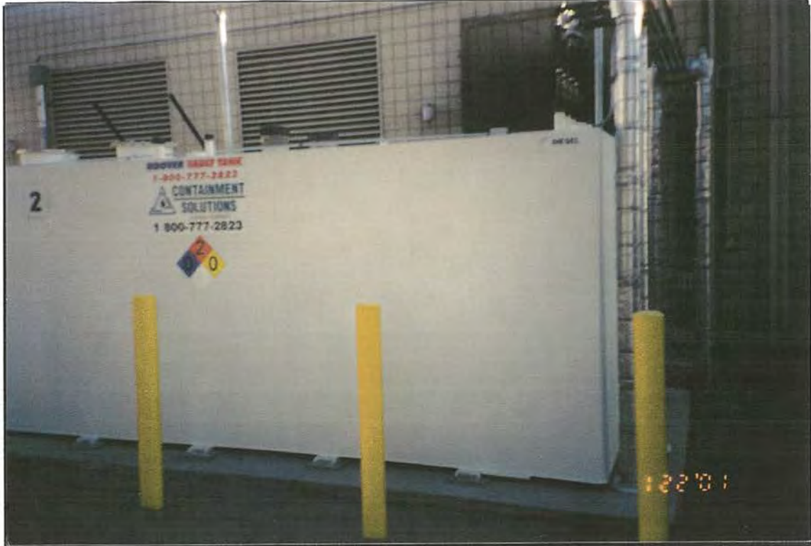
Generator #2 Fuel Tank B5
