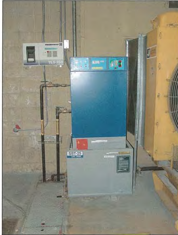
Generator #2 Day Tank B6
